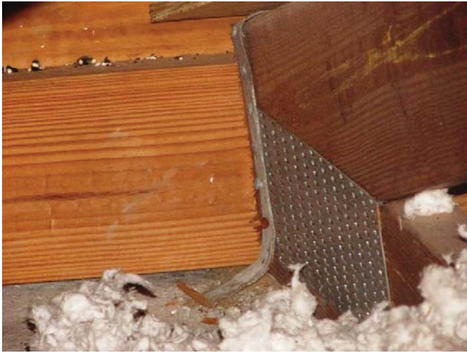
Toe Nail; over 1/2" gap from truss
