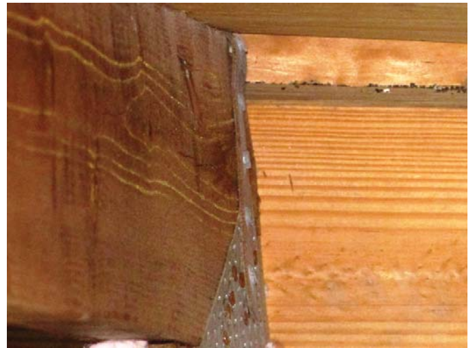
Toe Nail; over 1/2" gap from truss (other side)
