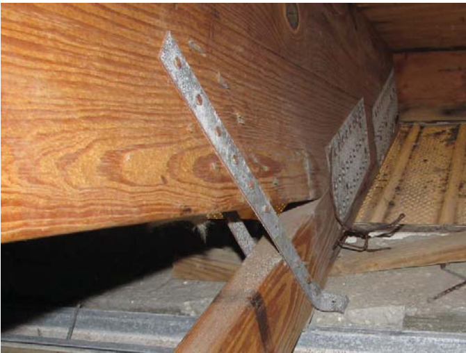
Toe Nail; over 1/2" gap from truss
